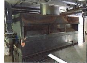
Swim Center Boiler
